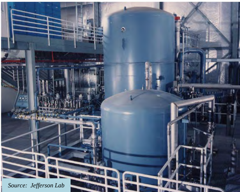
Figure 2-5 Typical Cryogenic Plant Equipment (Cold Box)
