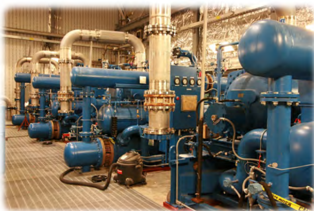
Figure 3-10 Cryogenic Plant Compressor Room
